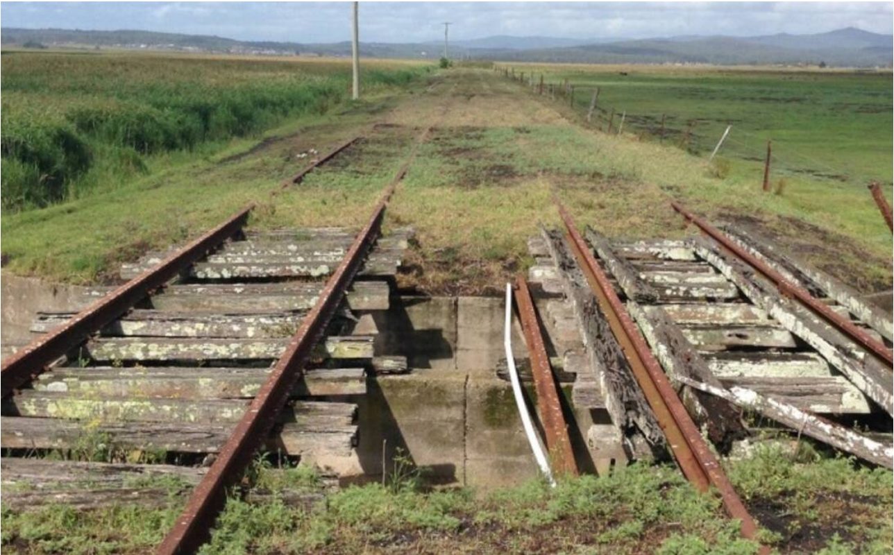
PROGRESS: The Richmond Vale Rail Trail presents an exciting opportunity to open up the stunning Hunter Wetlands National Park to the public.
