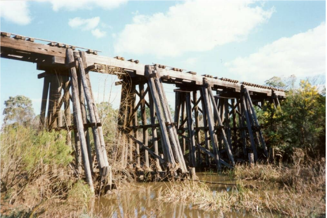
IN DECAY: The Wallis Creek timber trestle bridge on the old abandoned Richmond Vale Railway (RVR) line.
