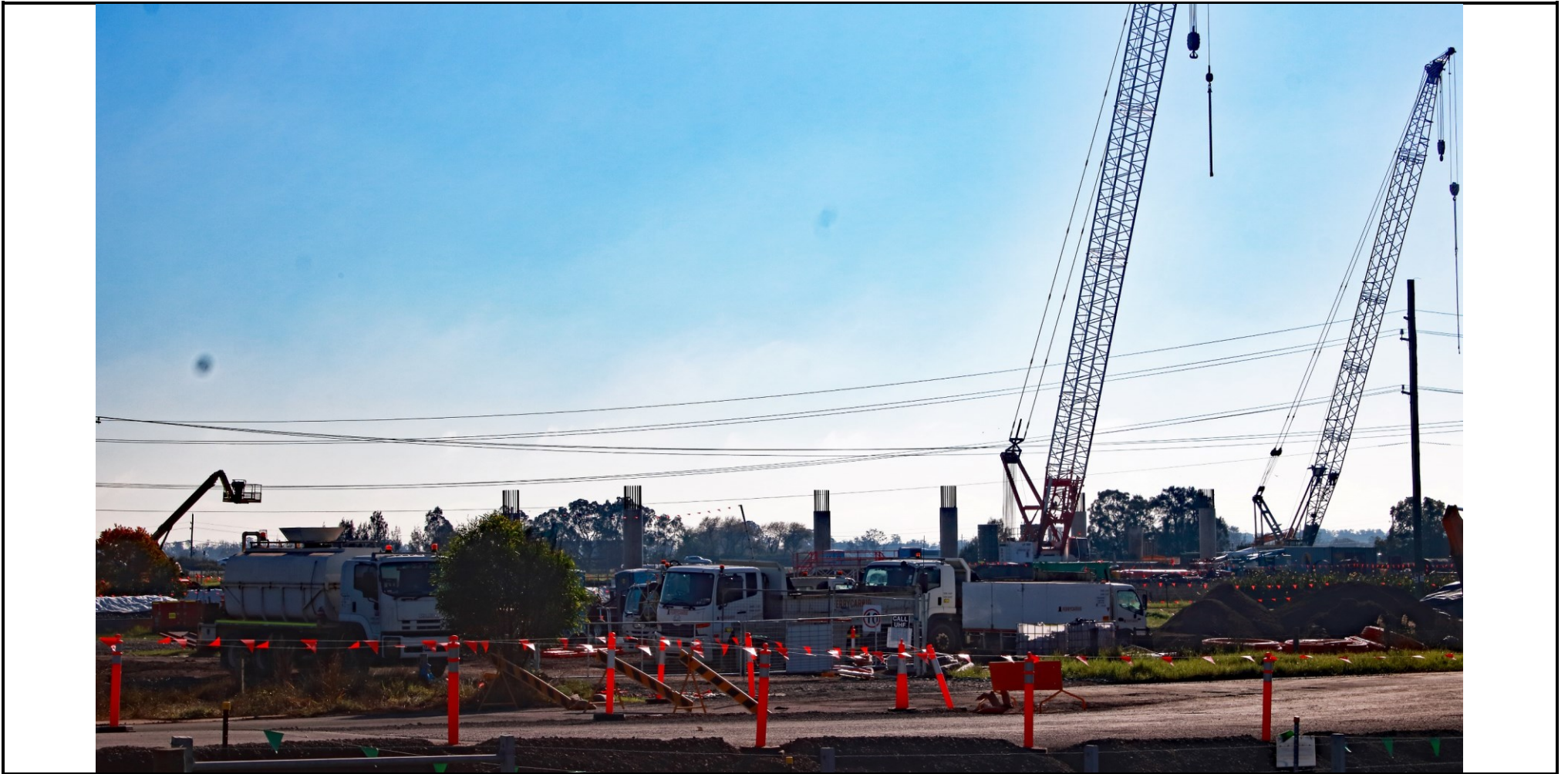
Picture 7: Bridge Piling Activities associated with Viaduct East of Re-located Aurizon Access Road (Tarro) – May 26th 2024.
