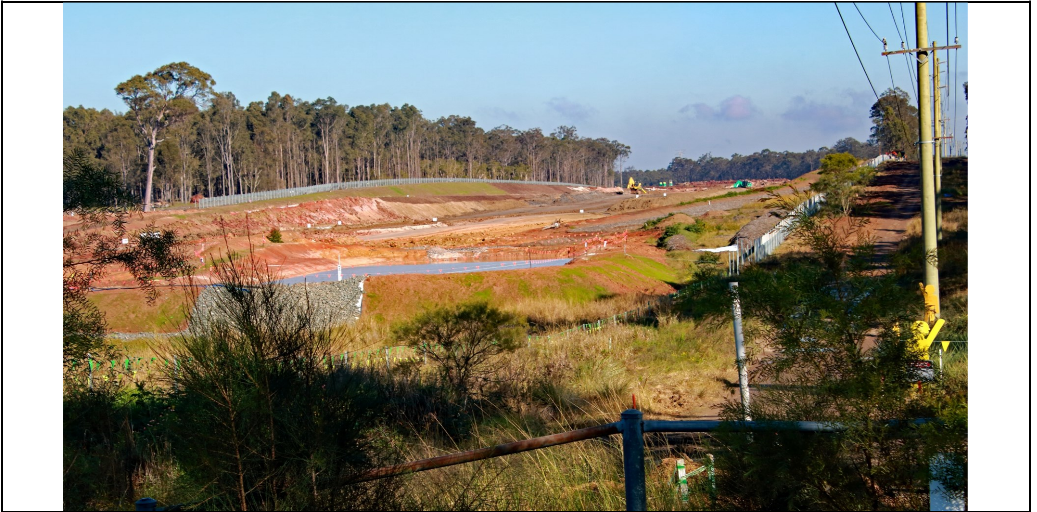
Picture 4: Progress on Black Hill to Tarro Section of M1 Extension – May 26 th 2024.
