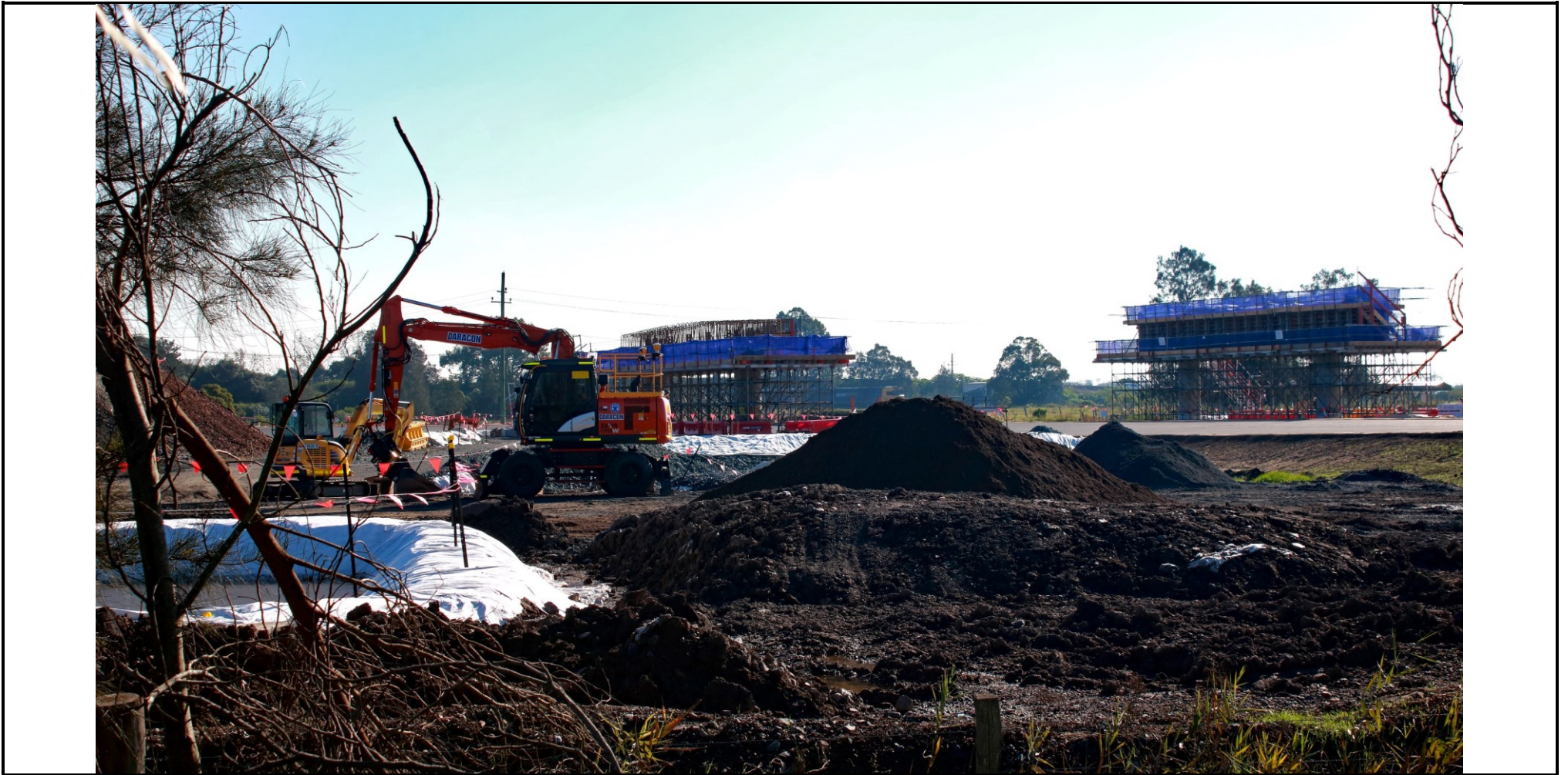
Picture 5: Near Re-located Aurizon Access Road Section of M1 Extension (Tarro) – May 26th 2024.
