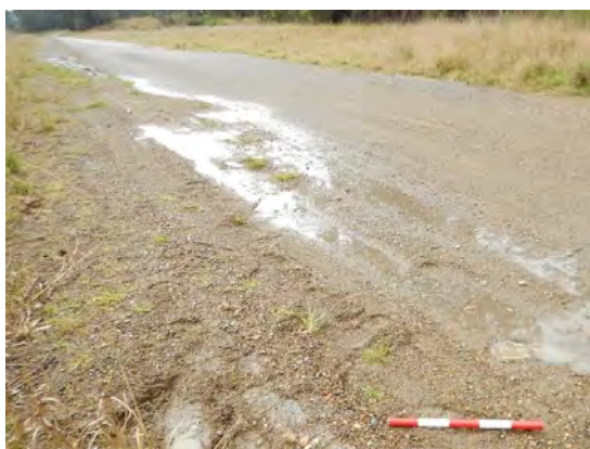
Figure 133: Imported road base and gravels on Seahampton Road and adjacent road shoulder, east aspect
